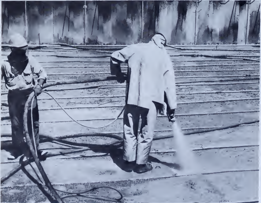
Figure 121.—Final sandblasting of construction joints at Glen Canyon Dam, in Arizona. This is an expeditious and effective means of construction joint cleanup. P557-420-05101.
